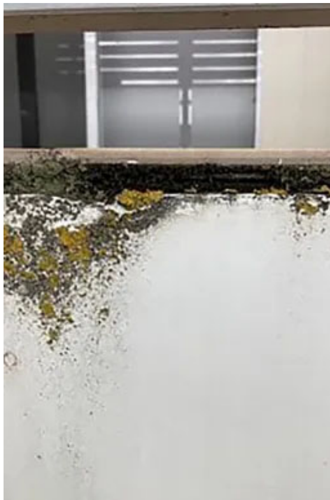
Water ingress to balcony. CLADDING SAFETY VICTORIA
