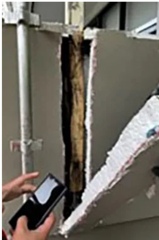
Timber framing to balustrade rotten from water ingress. CLADDING SAFETY VICTORIA
