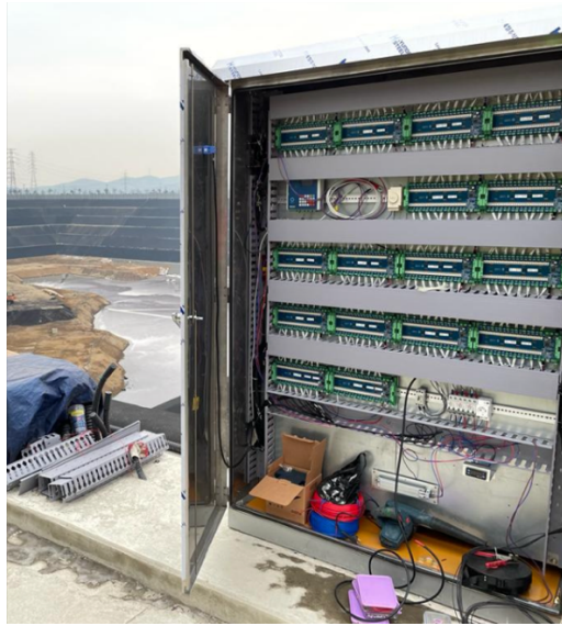
Case Study 1 - eFix automatic monitoring box during installation
