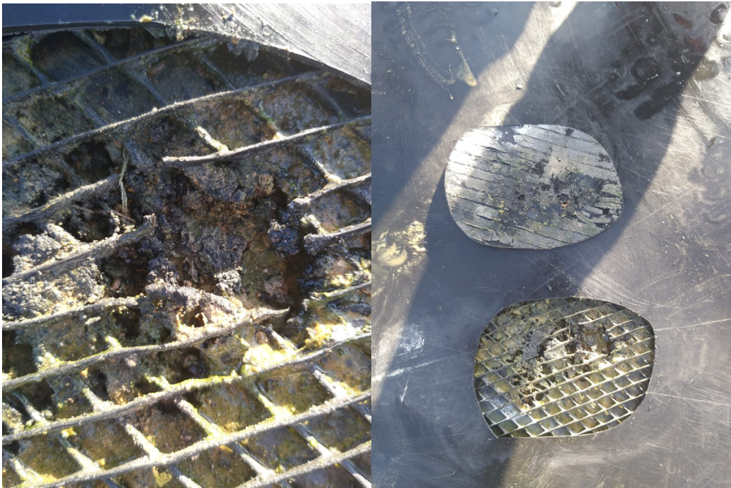
Case Study 2 - fire damage discovered using eFix technology
