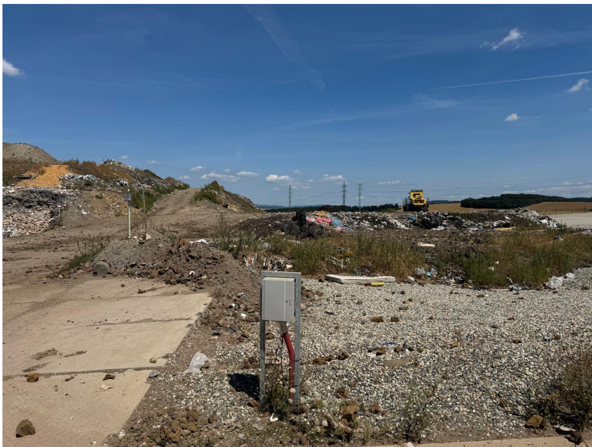
Case Study 2 - completed offline eFix a monitoring box on a landfill site
