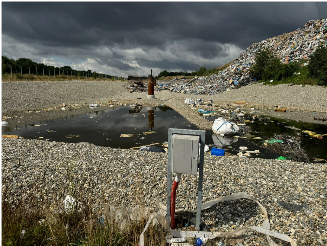
eFix Monitoring Box at a Landfill Leachate Pond
