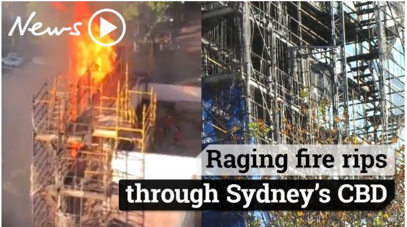
Plumes of black smoke have billowed across Sydney’s CBD from a large building fire on Macquarie Street.
