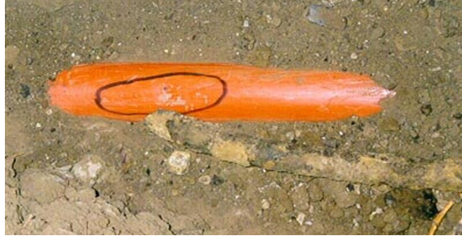
Figure 2: External Crack from Long-term Third-Party Stress [76]
