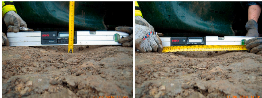
Fig. 7. Macro irregularities and depressions on the slope surface.
