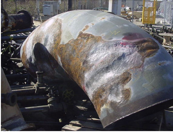
Figure 17.3 Corrosion under insulation on inorganic zinc pipe section.
