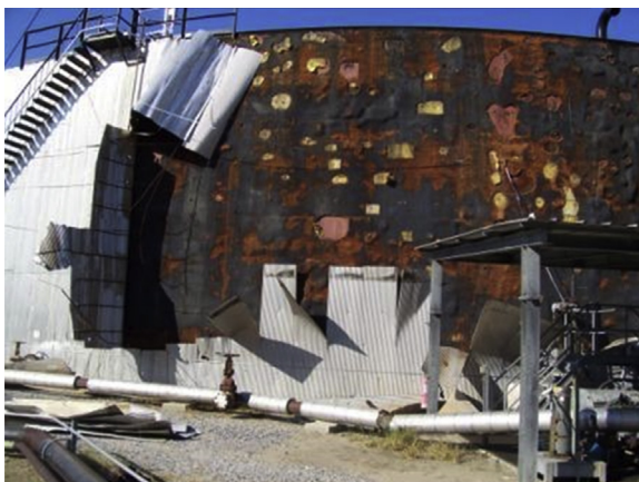
Figure 17.2 Corrosion under insulation on Naptha tank.
