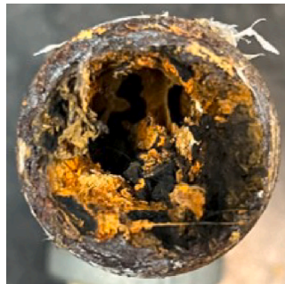
Fig. 19. Example of a blocked pipe due to depositions.
