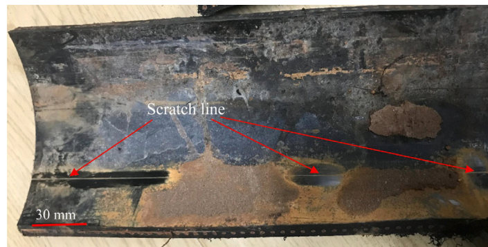
Fig. 15. Example of inner surface wear damage in a 6-year-old in-service steel wire-reinforced composite pipe [79].
