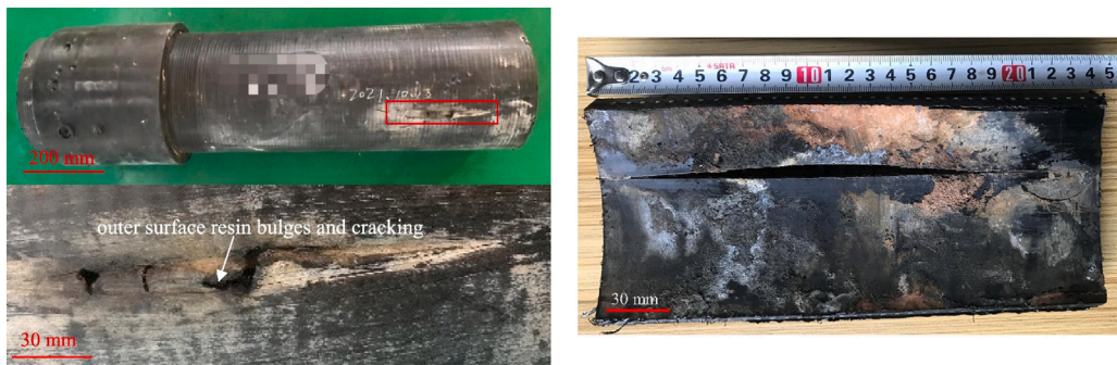
Fig. 14. Steel wire-reinforced composite pipe sample after 6 years of service with a crack [79].
