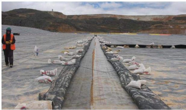
Figure 8.4: Separation by shrinkage in two panels of GCL installed
