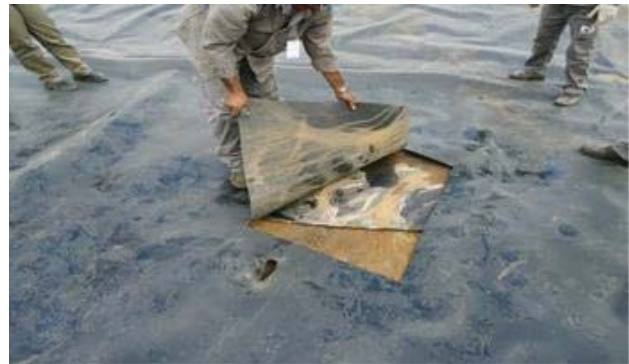
Figure 8.21. Exhumation of HDPE samples – FBM Security dike (Santos, 2016).
