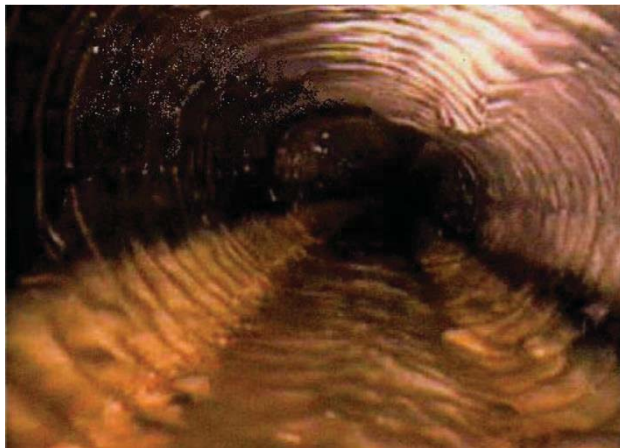
Figure 8.15: Interior of a solution collection pipe below a heap leach pad
