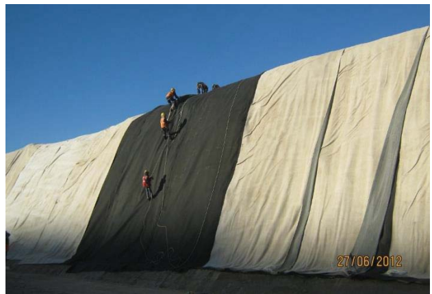
Figure 8.7: Installation of geocomposite for protection (black) and GCL (white) on an almost vertical slope
