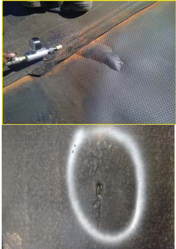
Figure 7.5. (a) Separation in-plane for a geomembrane having 0.9 mm micro-spike height and (b) Geomembrane manufactured with discontinuities including ridges and holes installed despite the designer's specification requiring a 0.9 mm micro-spike height and minimum thickness of 1.5 mm.
