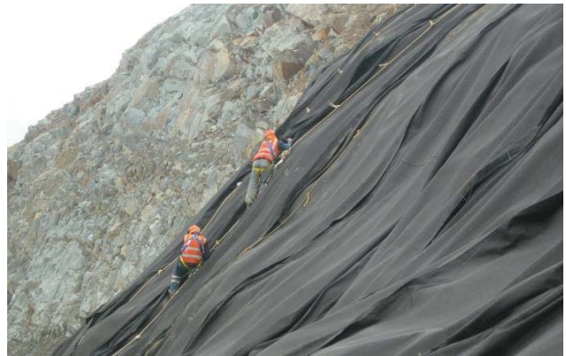
Figure 8.6: Typical protection with heavy geotextile (upper) and geocomposite (lower) for geosynthetics installation in difficult slopes
