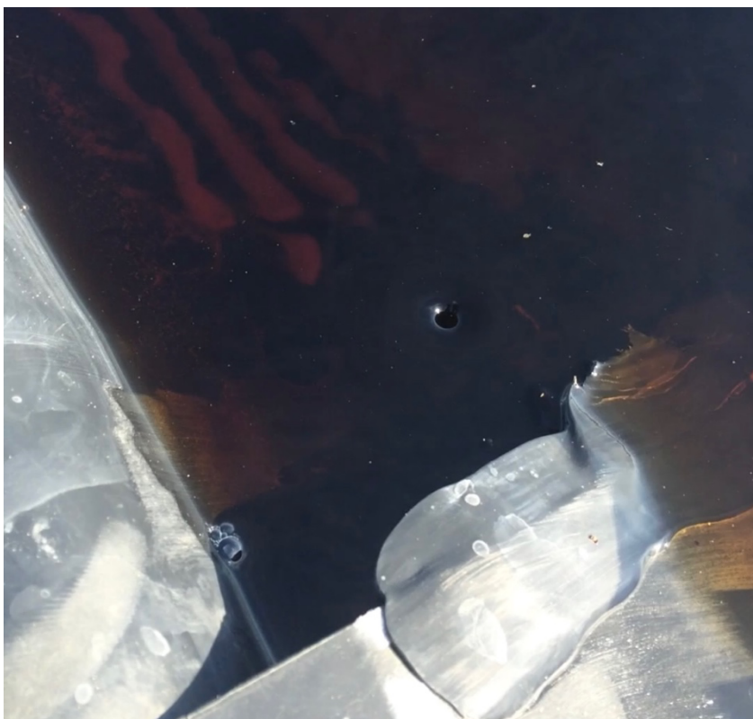
A torn weld hole with a liquid vortex as it flows through the hole.
