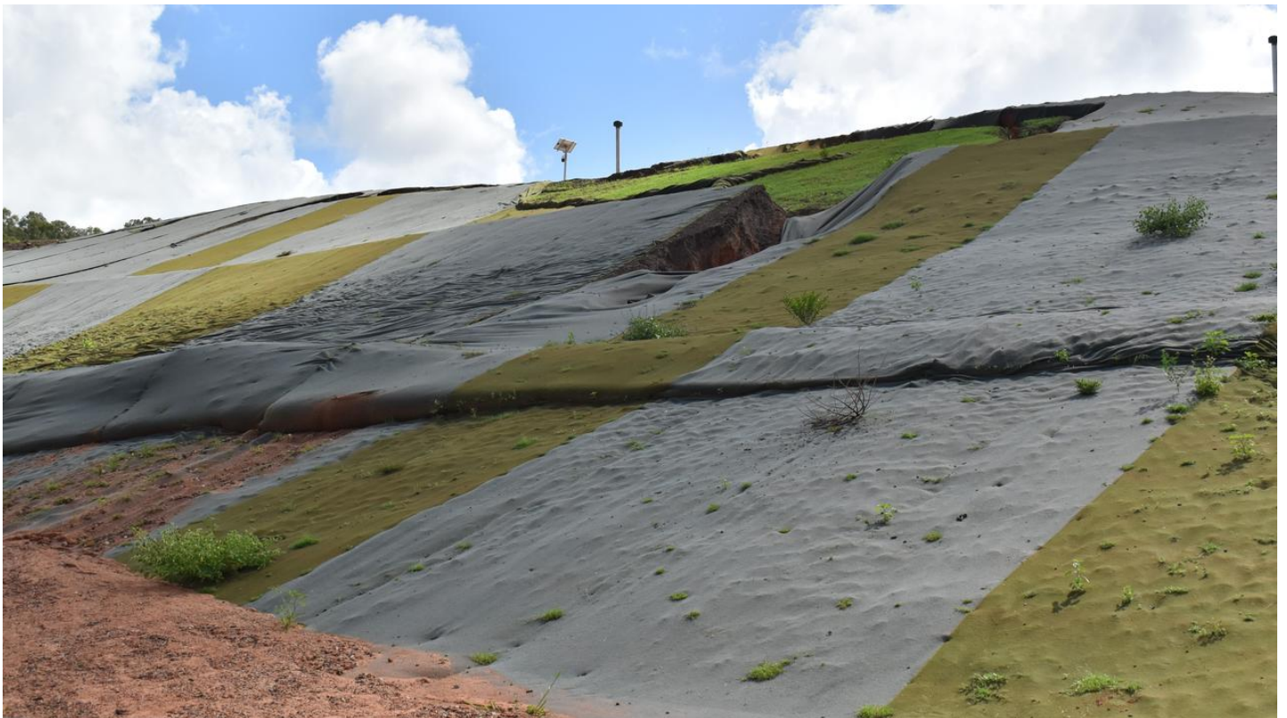
The costly works at the oldest part of the dump, pictured, have slumped at the top of the capping program. Picture: Cameron Bates
