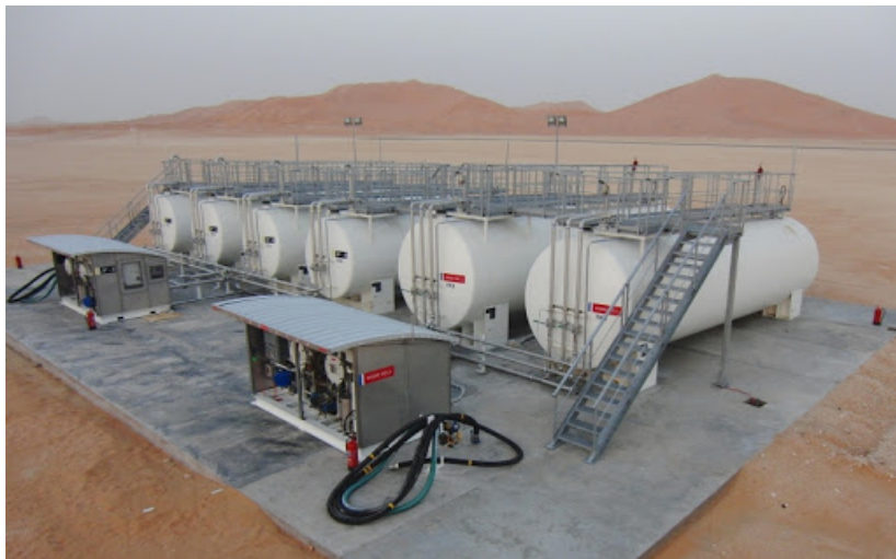
Figure 3. Bund Liner and Pad for Temporary Diesel Storage and Refuelling Facility in Conflict Zone
