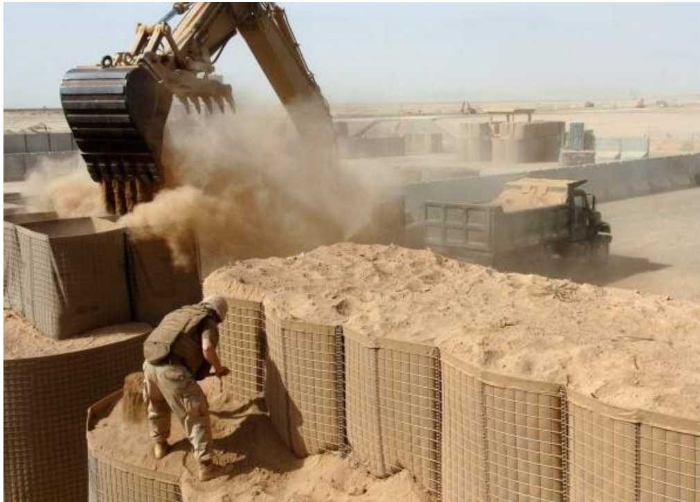
Figure 4. Sand-Filled Gabions being Filled with Sand. Gabions are used as military fortifications for protection against enemy fire and mortar attacks. Sand-Filled gabions can be installed and deployed quickly wherever needed. They are widely used today in military bases especially for protecting soldiers in mess halls and sleeping quarters.
