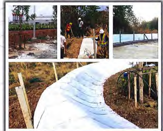
Application : Berm Reference Site : Berm for Flood Protection at Nong Kae industrial estate, Saraburi
