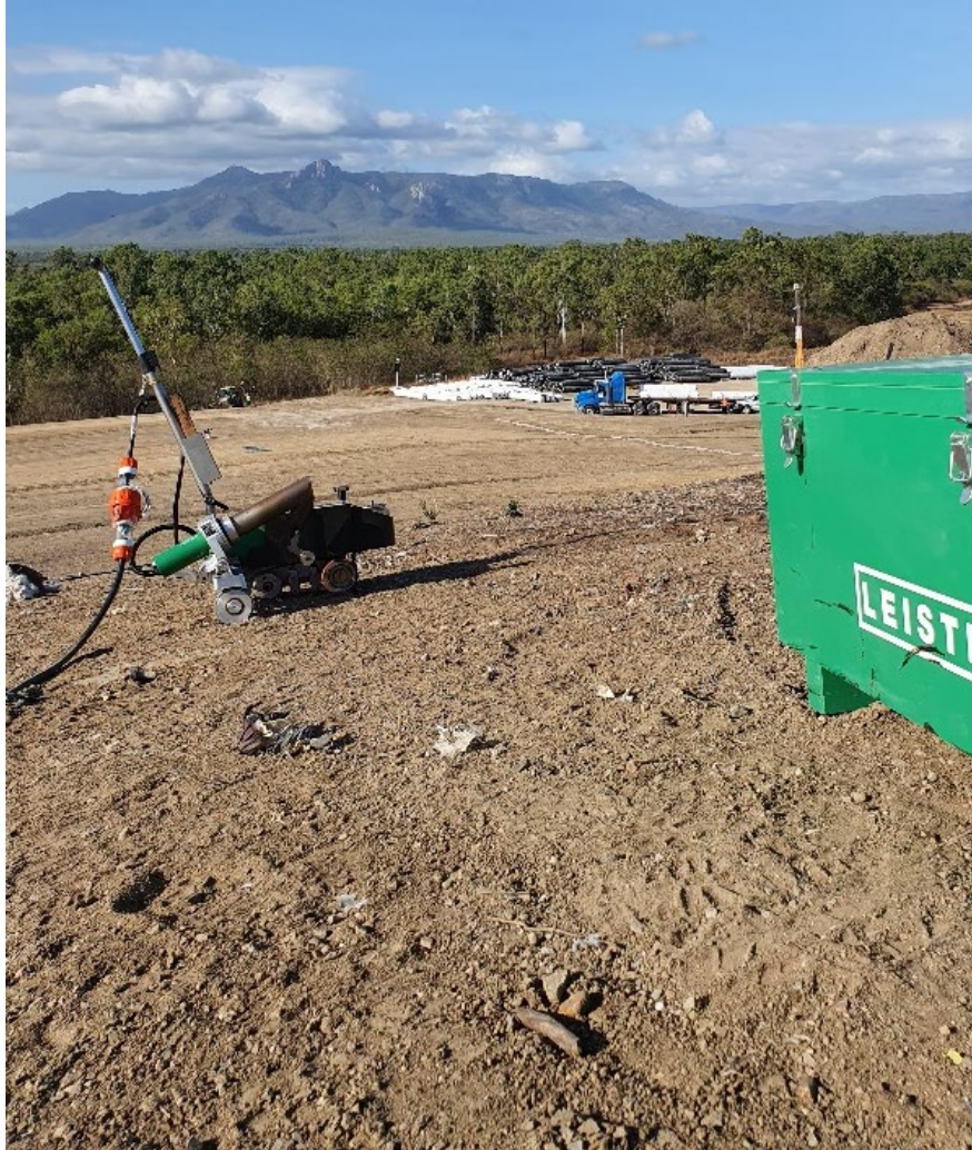
Figure 1: When a rough subgrade must be capped without using a gas torch, then Coletanche BGM with electric welding is the solution
