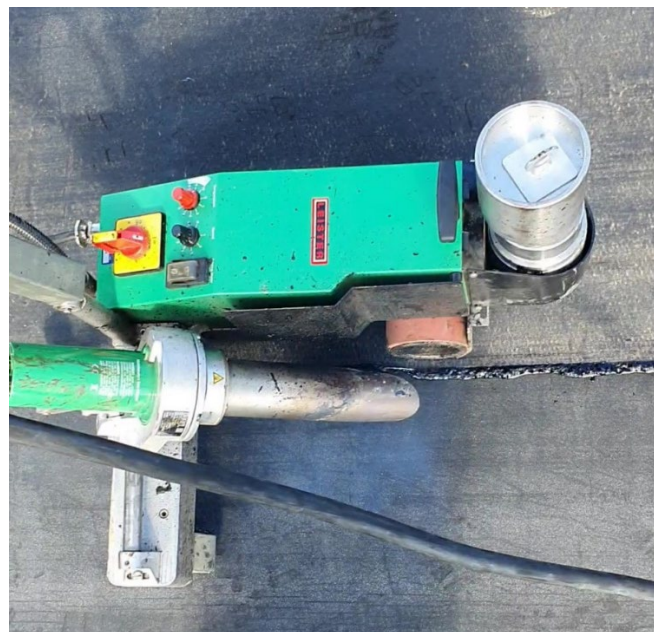
Figure 9: An overhead shot of the hot air welder in operation reveals a consistent weld and bitumen beading
