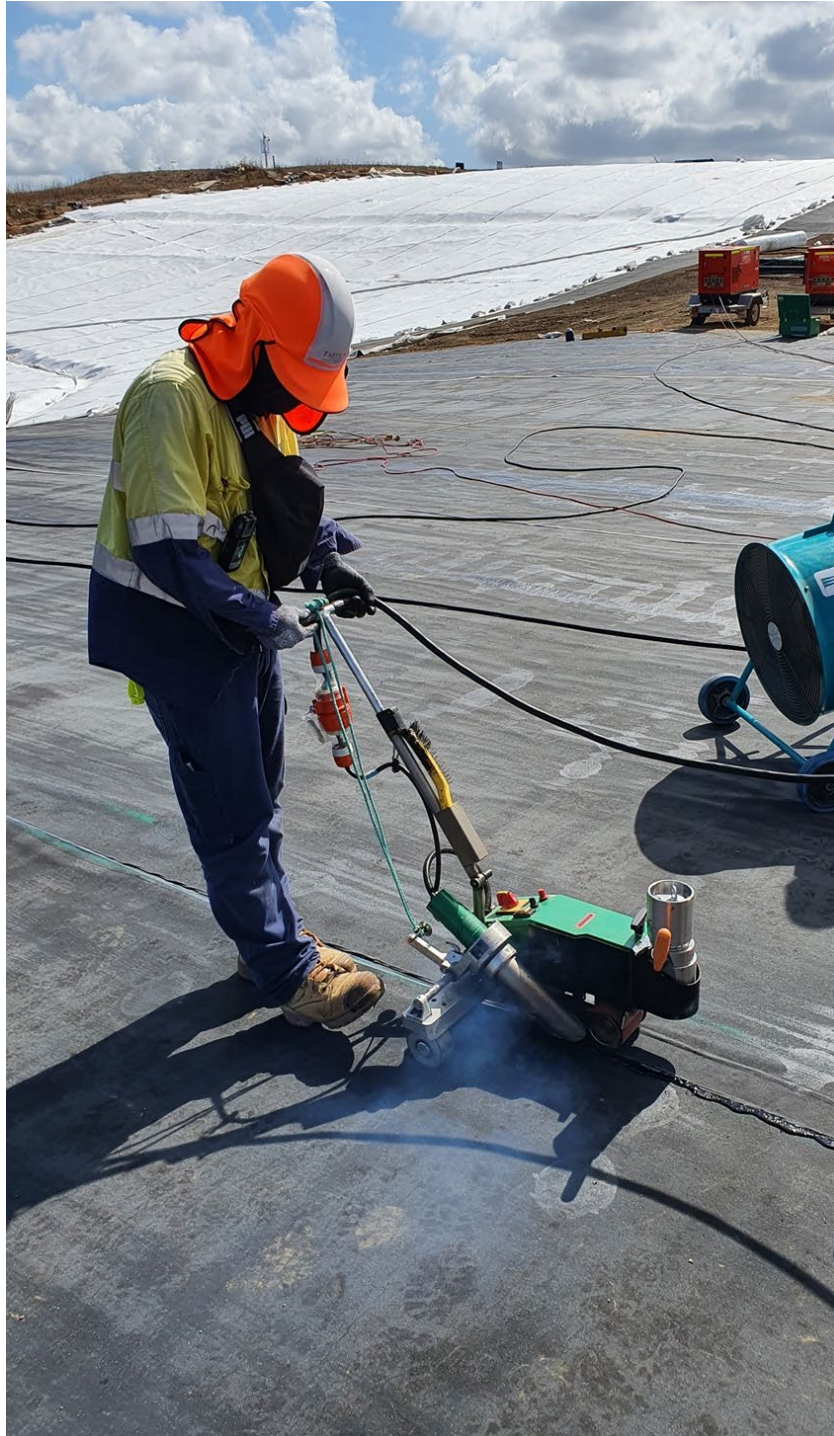
Figure 5: Good seaming is shown taking place in the foreground and the rough subgrade is shown in the background. Also shown in the background is the white drainage geocomposite placed on the Coletanche.
