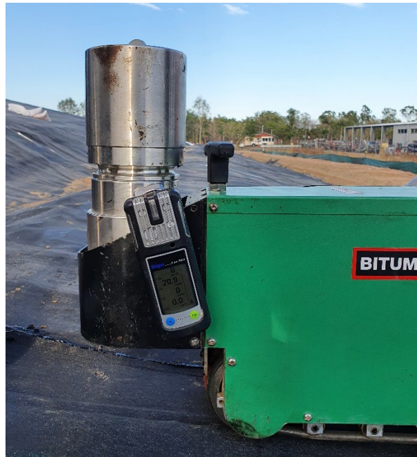
Figure 8: Methane Gas detection monitors were mounted directly to the welder as an extra safeguard
