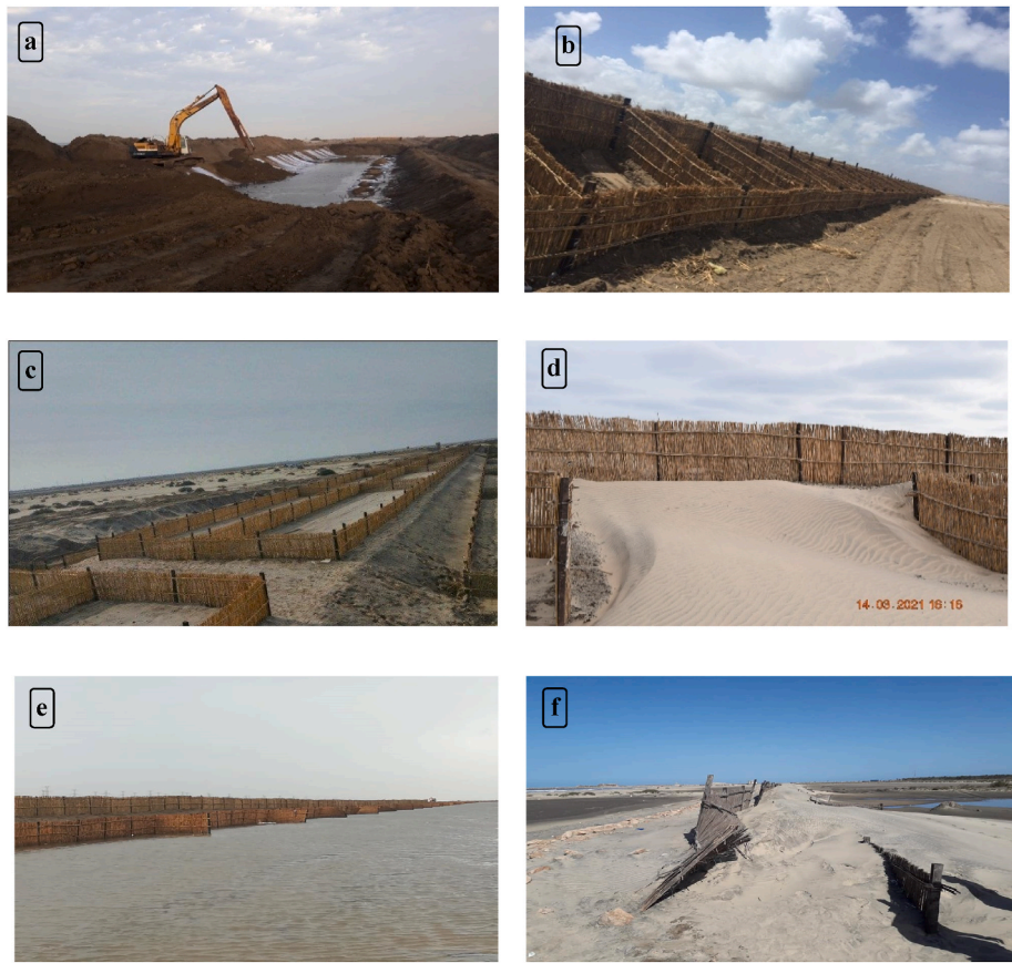
Fig. 6. Construction phases of the artificial sand dune (31°29'49.93"N, 30°41'15.74"E); a) Geotextile layer and the clay layer (the core of dune); b) and c) Sand bumpers installation and the sides and top dune; d) trapped sands induced wind; e) and f) Observed impacts due to inundation and rough weather.
