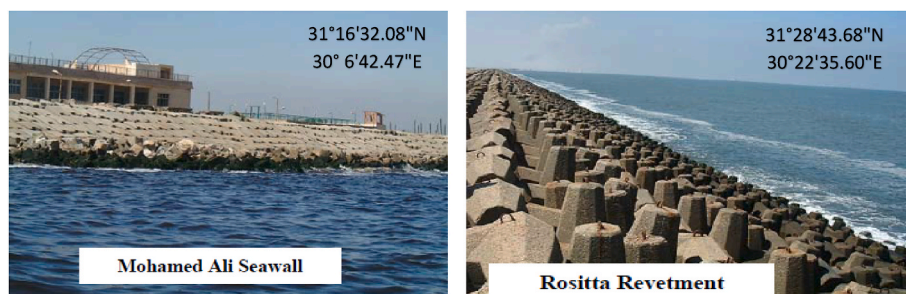
Fig. 3. Examples for the implemented hard structures as a protection adaptation option to SLR (Iskander, 2010); Left panel: Mohamed Ali Seawall implemented at Abo Qir bay; Right panel: Revetment located at Rosetta city, Nile Delta, Egypt.
