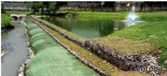
Picture 1: Golf Course Stormwater Protection (before)
