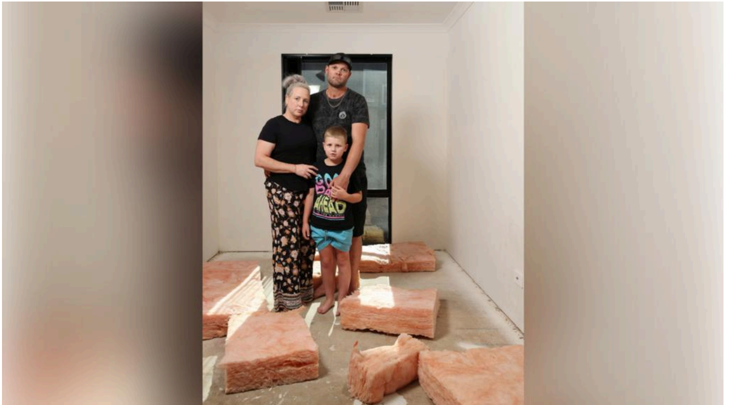
Thousands of WA homeowners were impacted by the defective Iplex pipe saga. Pictured is Chris and Sarah Lyne with their son Nate in one of the damaged rooms. Credit: Daniel Wilkins/The West Australian
