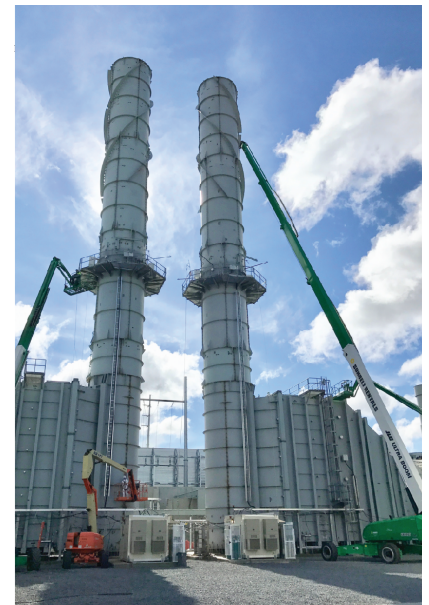
Shop-primed with zinc in advance, the 185-foot-tall stack structures were delivered from overseas and erected prior to surface preparation, spot-priming and coating application. Cranes and lifts were utilized throughout the project to apply coatings at heights exceeding 185 feet.
