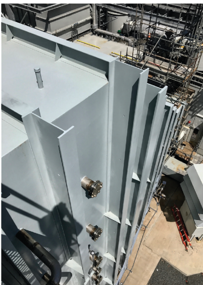
Nuts and bolts and tight angles required brush and roller application to ensure full coverage.
