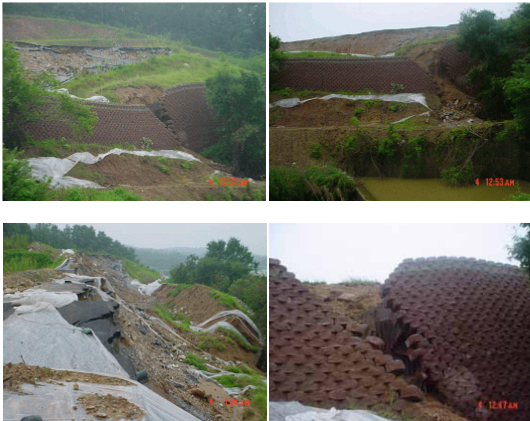
Figure 1. Photos taken after the collapse
