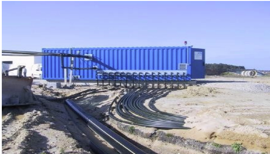
Fig. 3. LFG manifold pipe system for gas collection at dumpyards Fig. 3. landfilled gas collection and manifold system at dumpyards.
