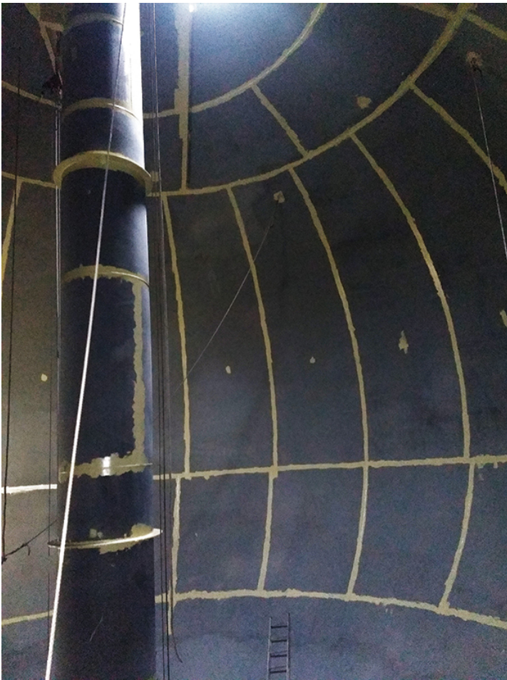
Figure 3: Applicators blasted the tower's interior to a Near White Metal standard, applied a zinc primer to the entire interior and then applied a stripe coat of the lining system to weld seams and edges to ensure full coverage of these hard-to-coat areas. A full coat of the 100%-solids, glass flake-reinforced lining followed. Courtesy of Sherwin-Williams Protective & Marine
