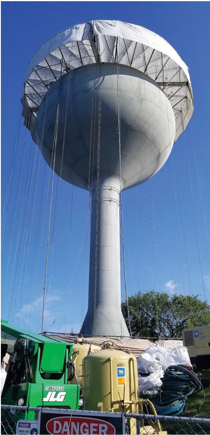
Figure 4: The coating contractor installed a full containment system around the tower to prevent dust, debris and coating overspray from escaping the job site during restoration work. Courtesy of Sherwin-Williams Protective & Marine
