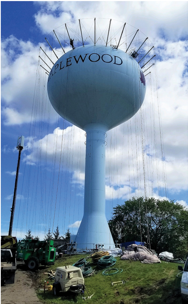
Figure 2: The water tower's exterior had faded and was in need of a refresh to liven up the image of the Maplewood, Minnesota, community. Courtesy of Sherwin-Williams Protective & Marine
