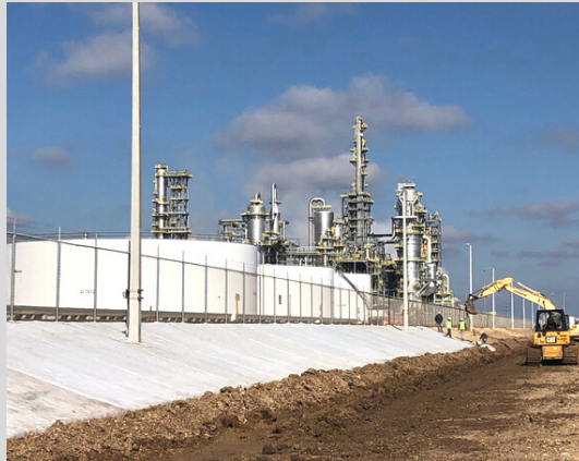
SLOPE EROSION Berm Protection
