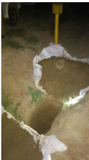
Figure 1: Digging detected and stopped on a pipeline in India.
