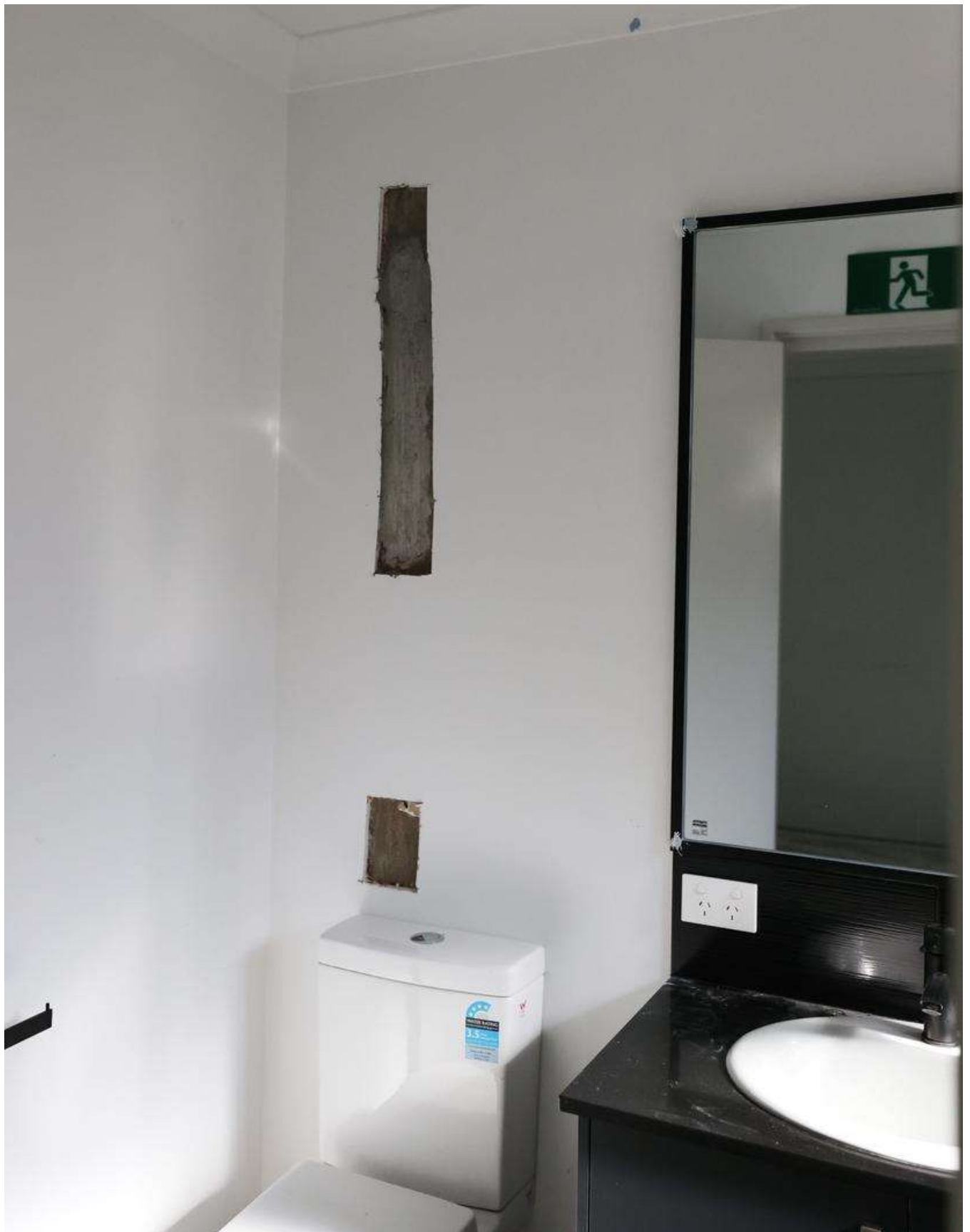
📷 Thousands of WA homeowners are impacted by the defective Iplex pipe saga. Credit: Daniel Wilkins/The West Australian
