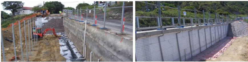
Fig. 3 Left the stabilised excavation with horizontal drain connected to a trench drain. Right the Geofoam remediation prior to shotcreting
