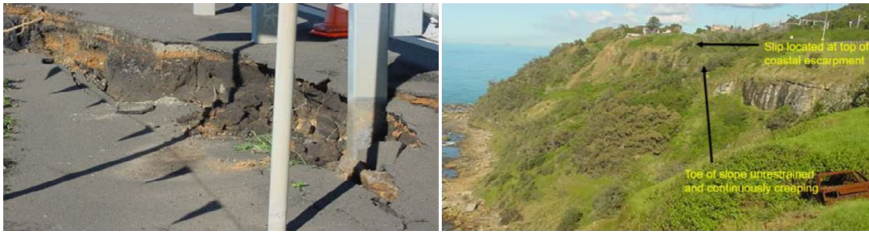
Fig. 2 Left the step in the pavement on the guardrail. Right slope location above cliff
