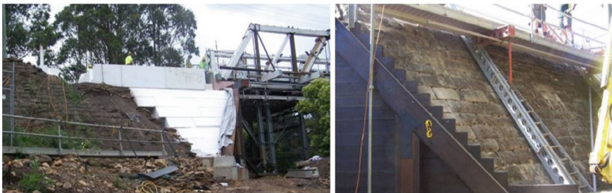
Fig. 5 The Geofram blocks placed prior to shotcrete, and the final remediation with the original drystone blocks reused
