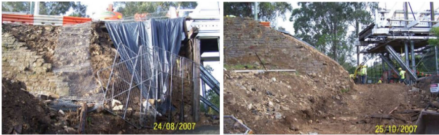
Fig. 4 Left the extent of the collapsed wing wall and drystone wall. Right the excavation and site preparation of placing the Geofram blocks
