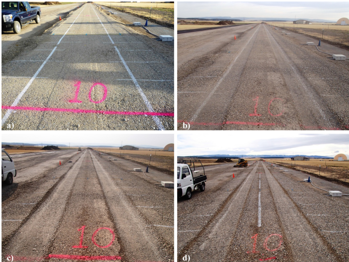
Fig. 6. Typical Phase II test section at (a) 0 mm, (b) 25 mm, (c) 50 mm, and (d) 75 mm of rut.
