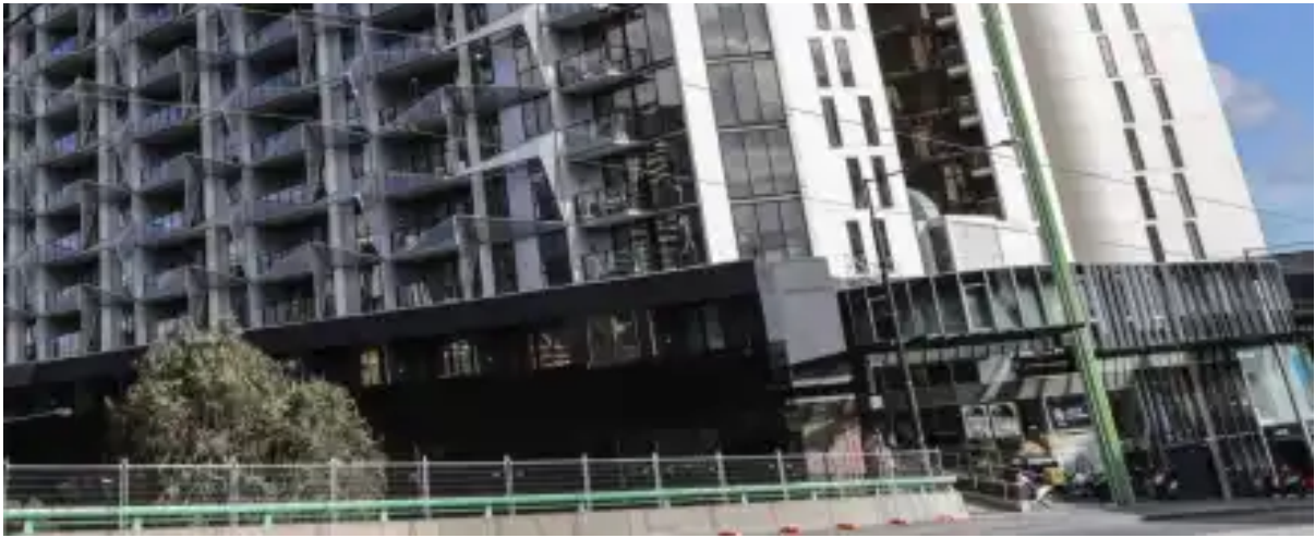
The cladding has been replaced but the question of liability is still in play at Melbourne's Lacrosse tower. Wayne Taylor
