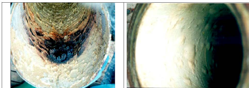
Figure 5. Chlorine degradation (left) and hydrogen chloride induced blistering (right) of a GRP pipe.
