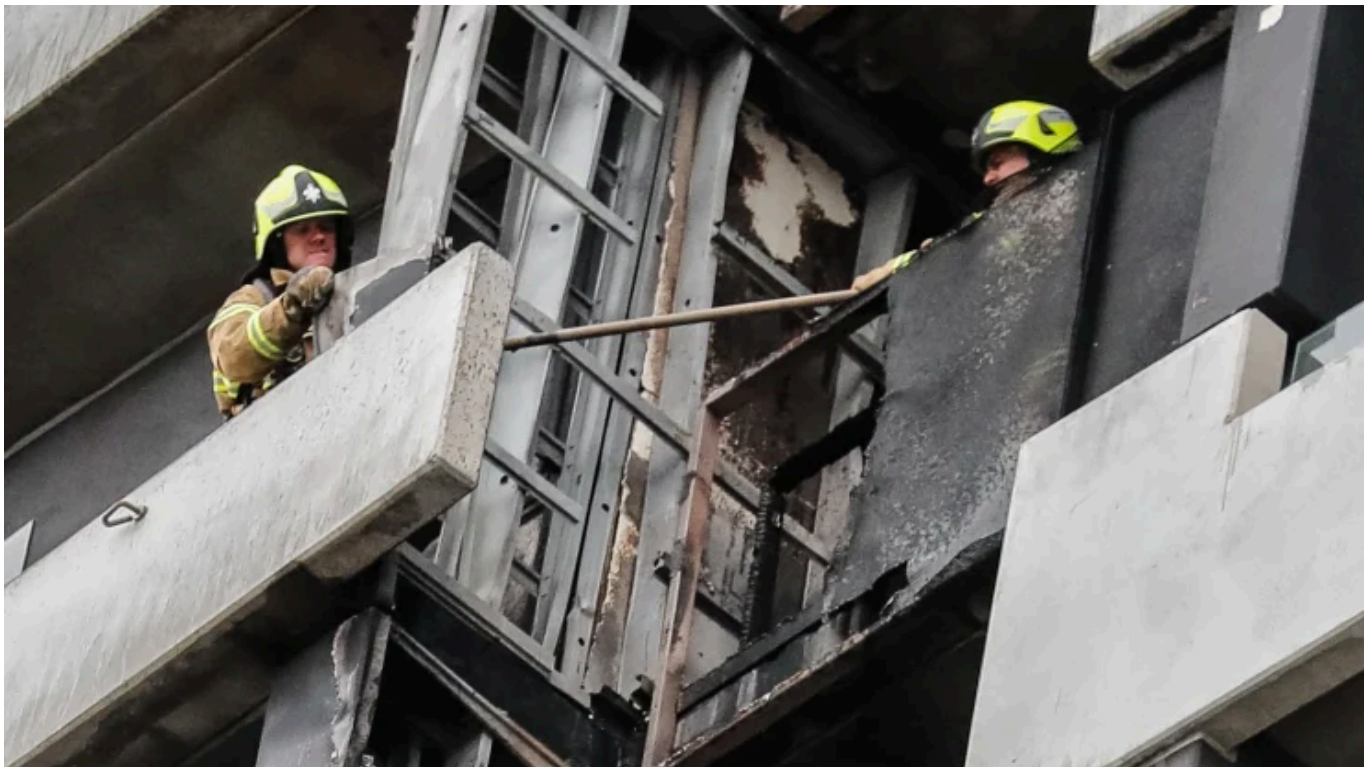
Firefighters inspect the damage at Melbourne's Neo 200 building in 2019. JASON SOUTH
