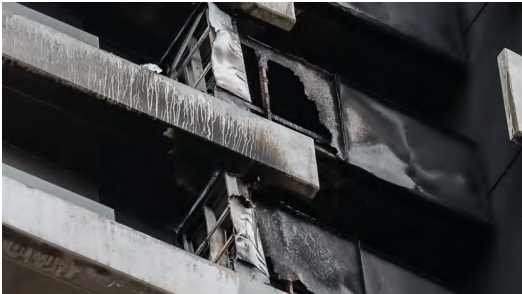
Cladding on a building in Spencer Street, Melbourne caught fire in November. JASON SOUTH
