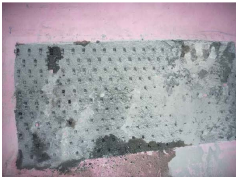
Figure 8. Typical Bulge Defect after Removal of HDPE
