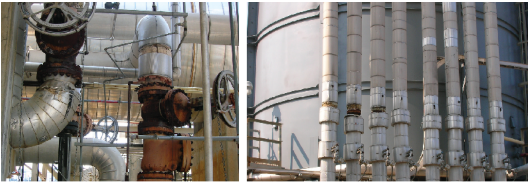
Fig. 3: Poor or unfinished installation, mechanical damage and signs of abuse during access are typical of aged insulation and jacketing in refineries and chemical plants. Evidence indicating a lack of CUI inspection and lack of maintenance on these easy-access feeder runs is clearly visible.
