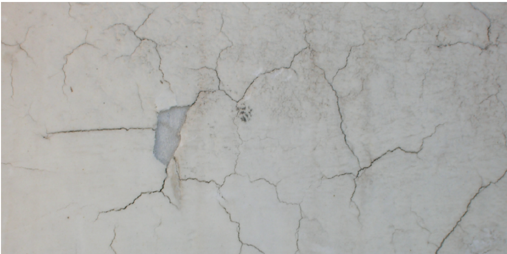
Fig. 2: This acrylic-spray-on insulation failed after two years from excessive film thickness or insufficient dry time between coats during application. The vessel may also have operated at temperatures beyond the acrylic resin's tolerance.
