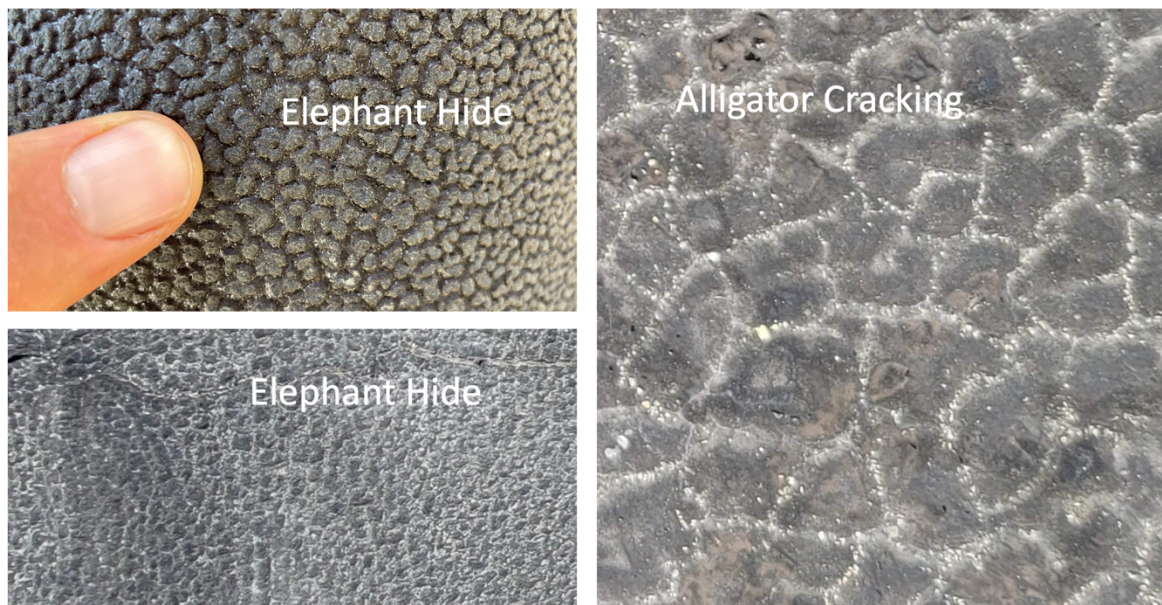
Figure 1. ‘Elephant Hide’ and ‘Alligator Cracking’ of Exposed and Heat Aged BGM
