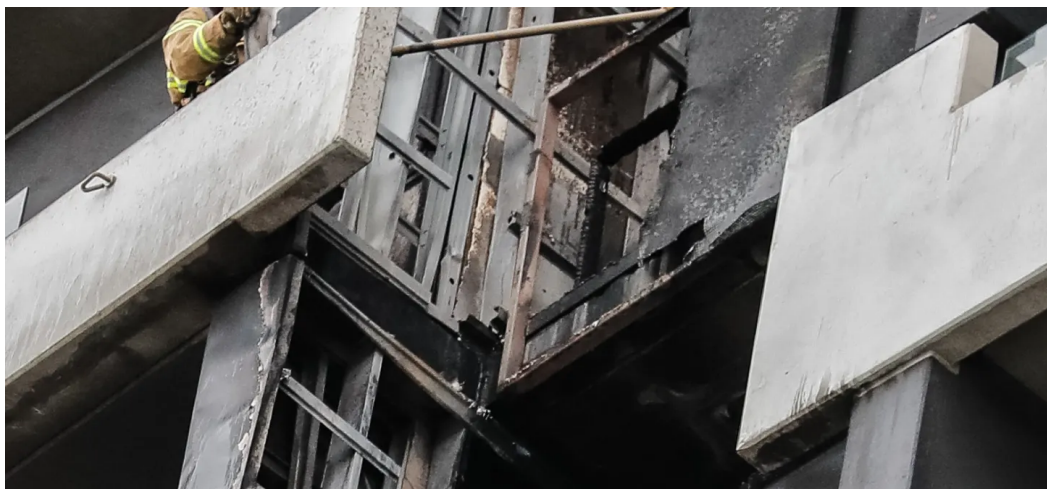
Firefighters inspect the damage at Melbourne's Neo 200 building. JASON SOUTH
