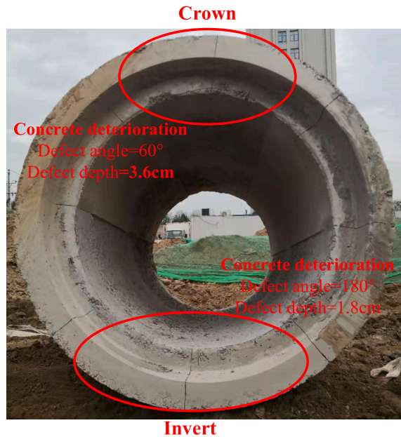
Fig. 3. The defected pipe.
