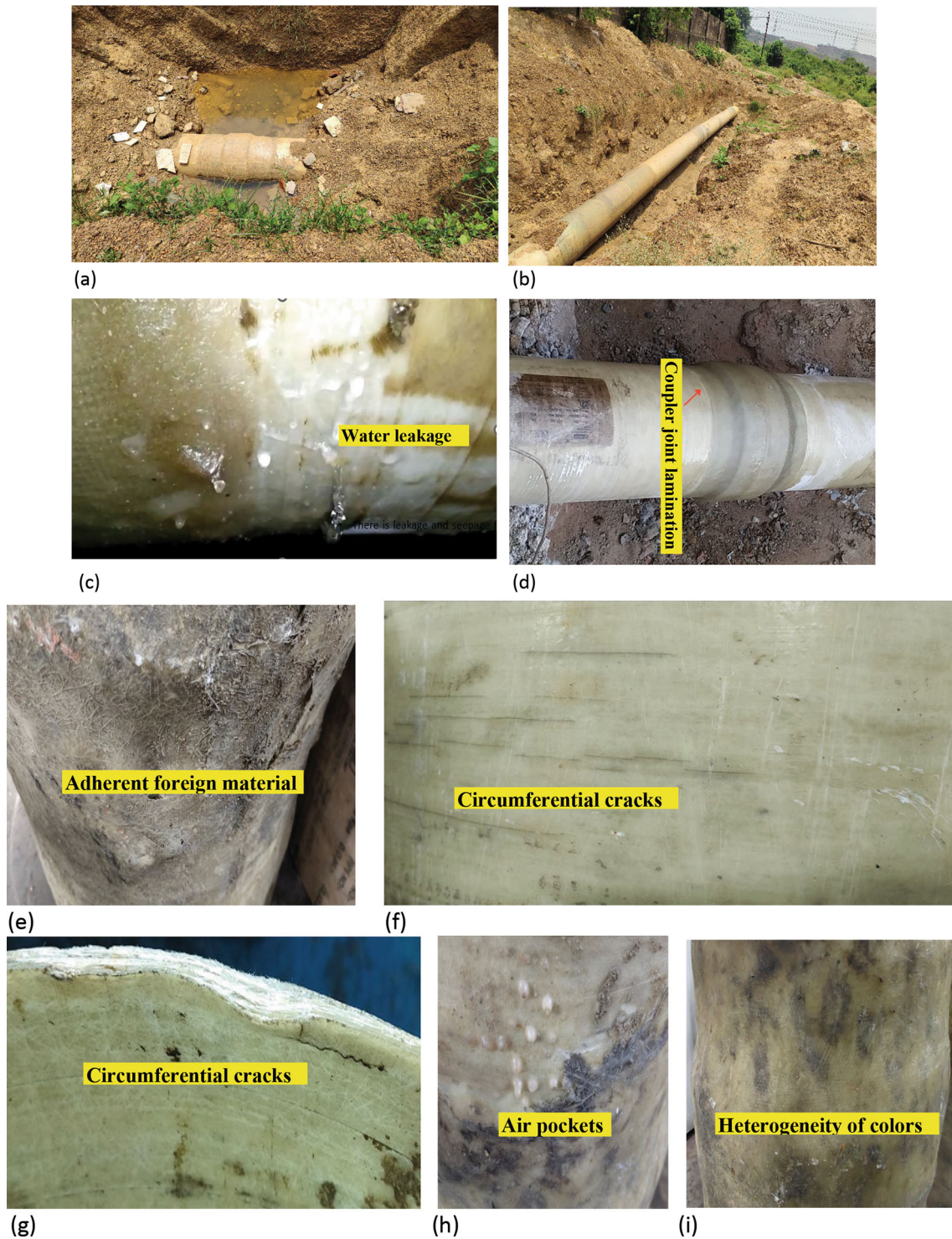
Fig. 2 (a, b) Site visit images at one of the locations (Graveyard) (c) Leakage through main pipe body (d) Coupler joint lamination where seepage was observed (e–i) Visual observations of unused pipe sample reveals abnormal features
