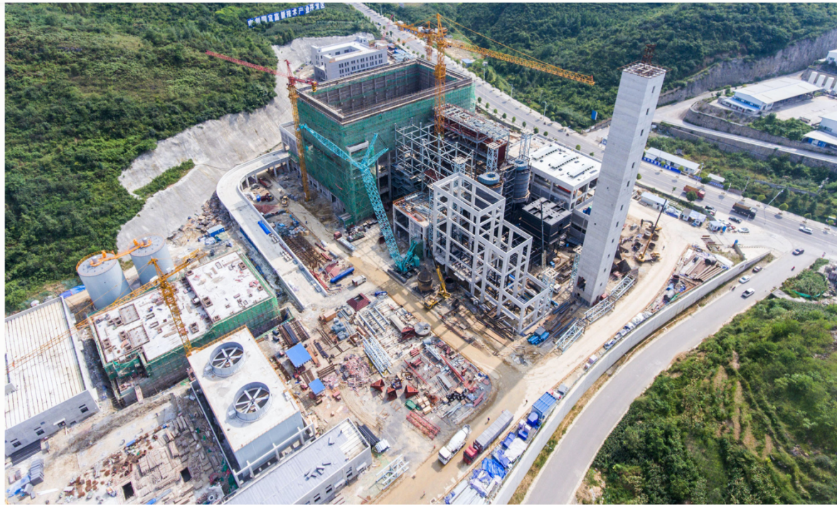
A waste-incineration power plant being built in Guizhou, photographed August 2019 (Image: Alamy)
