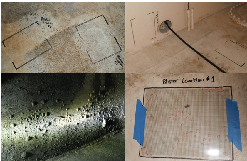
Fig. 3: Examples of blistering areas at first inspection
