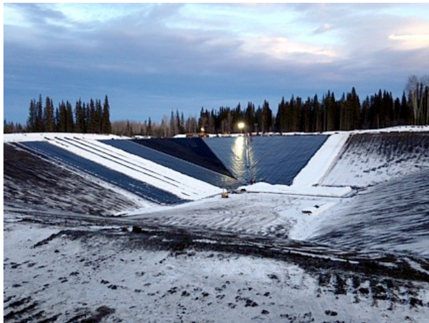
Figure 6. Installation under the lights.
