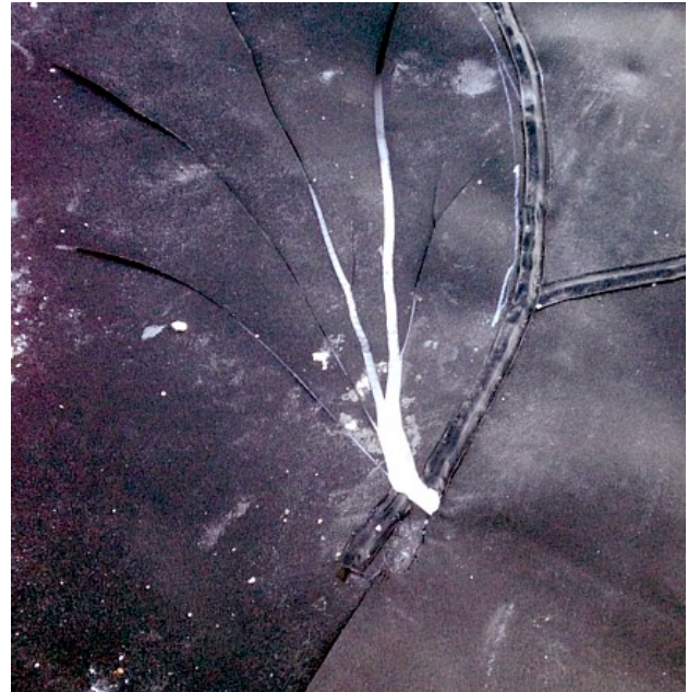
Figure 7. Cracking of the geomembrane.
