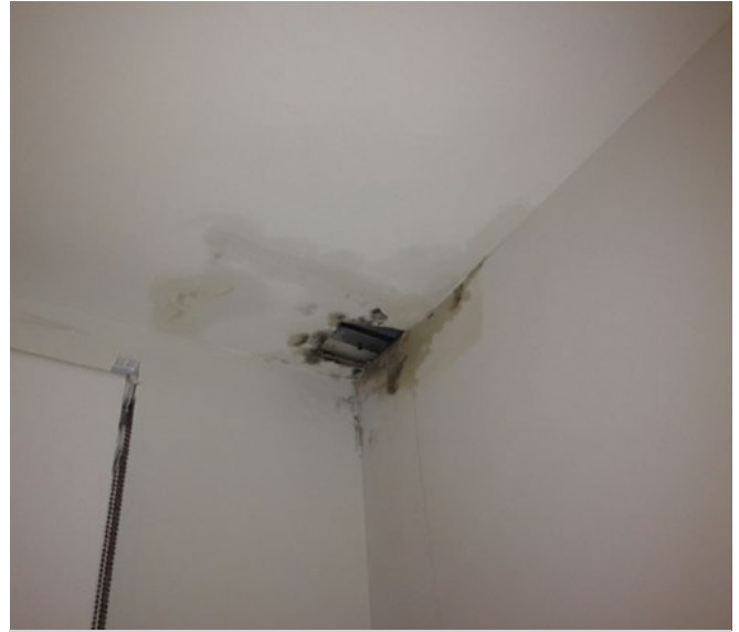
Moisture seeping through plaster walls.
