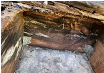
Figure 13. Example of insufficient or no waterproofing affecting a balustrade on a funded building in CSV's program (comprising 12 sole occupancy units)
