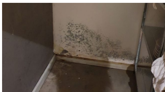
The presence of black mould on parts of the ceiling and walls in this apartment is extensive and widespread.
