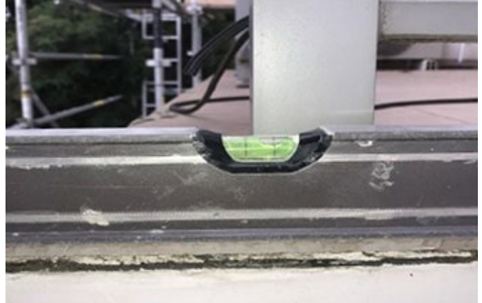
Balcony falling steeply away at edge.
