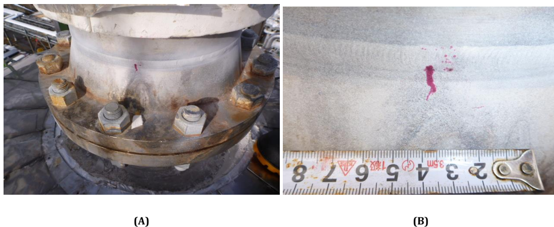
FIGURE 2: (A) SHOWS THE PHOTOGRAPH OF ECSCC AT TYPE 304L PIPE WELDS, (B) SHOWS ITS ENLARGEMENT
