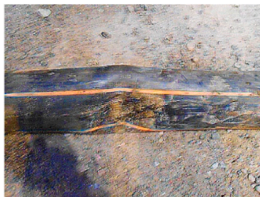
Fig. 4. The ductile failure of PE pipe subjected to mechanical excavation [27].
