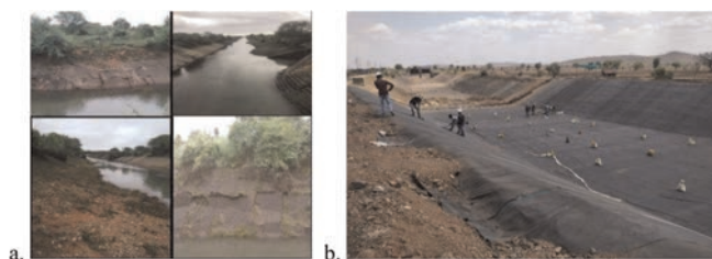
Figure 9. a. Irrigation canals in India – before / 9.b. Irrigation canals in India – during installation.
