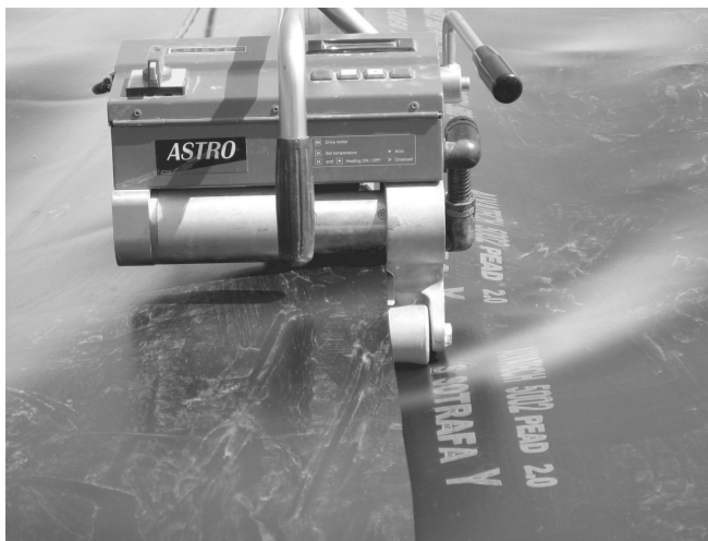
Figure 17.8 Photograph of seaming of HDPE geomembranes liners using a wedge welder (front view). Reproduced by permission of Sotrafa
