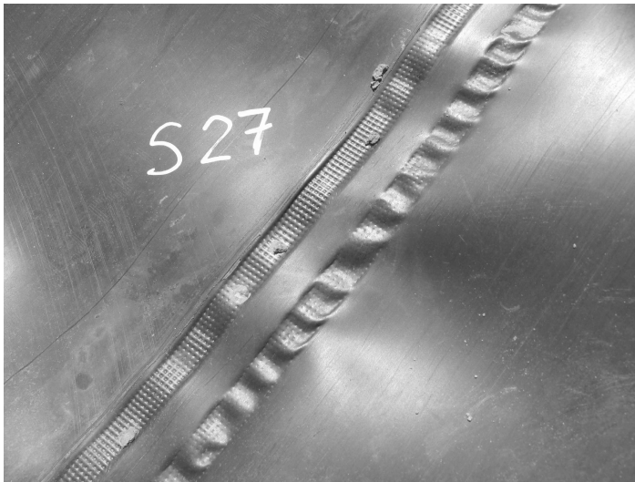
Figure 17.12 Photograph of weld tracks formed by hot wedge welding of 1 mm HDPE geomembranes. Note the poor tracking of the nip roller for the lower weld track
