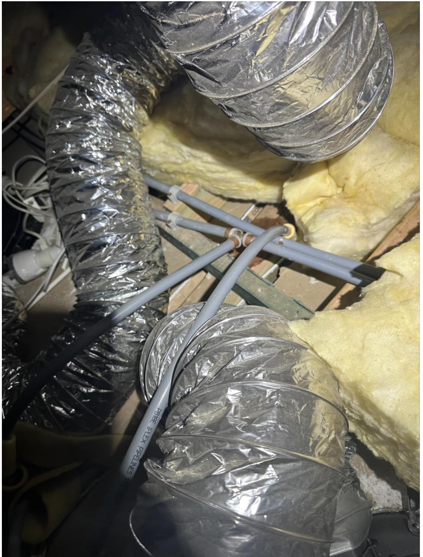
📷 Manufacturing defects in Pro-fit polybutylene pipes made by Iplex Australia and installed by BCG and Delstrat Groups. Credit: Supplied
