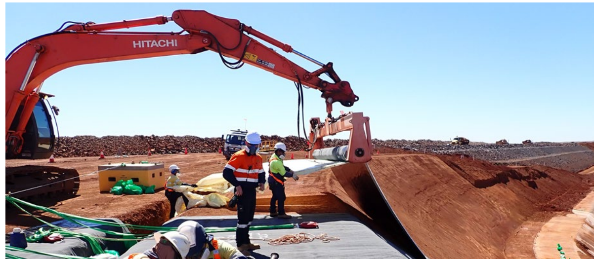
Unique hydraulically controlled installation equipment for Coletanche BGMs on extremely steep slopes. Western Australia
