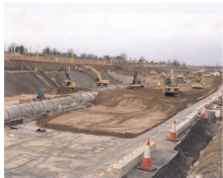
Figure 8b. Membrane over central collector.
