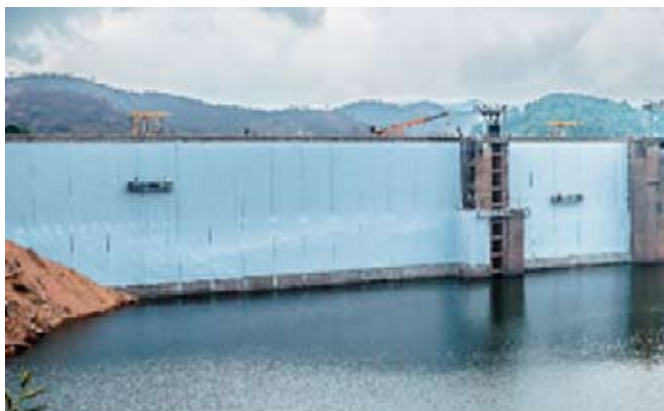
Fig. 8 : Overview of the dam with nearly 20% of the upstream face installed with Geomembrane system & Optical Fiber Cable.
