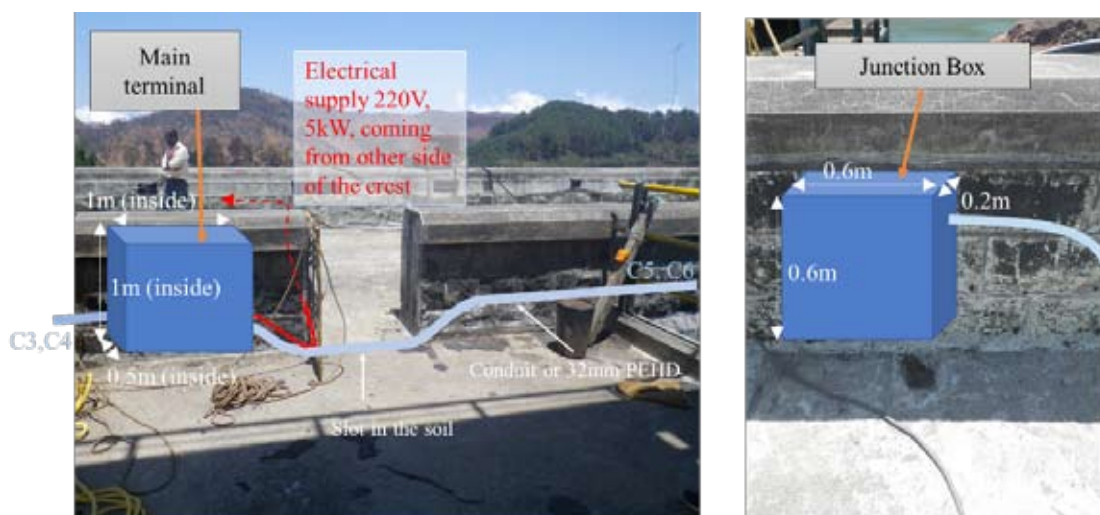
Fig. 9 : Shelter for Optical connections on the crest
