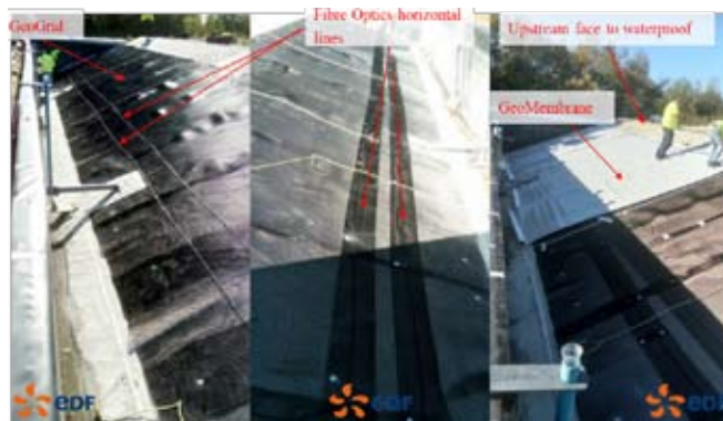
Fig. 4 : Cross section of the position of the fibre optics cable within the sandwich composed of the GM and the upstream face of the structure
