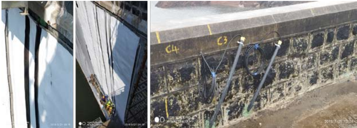
Fig. 10 : From Left to right, Fiber Optic cable positioned above the geotextile, geogrid protecting the fiber cable and an external protective pipe covering the exposed optical fiber cable at the crest
