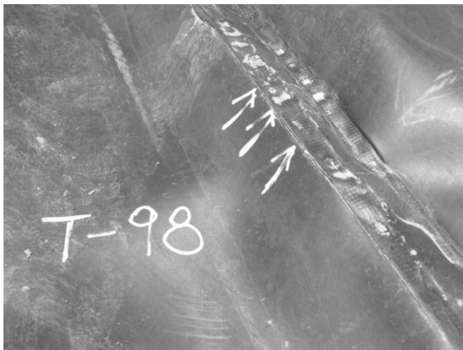
Figure 17.18 Photograph of a heat-affected weld in a 1 mm HDPE liner (note the buckling and distortion at the right side of the photograph)
