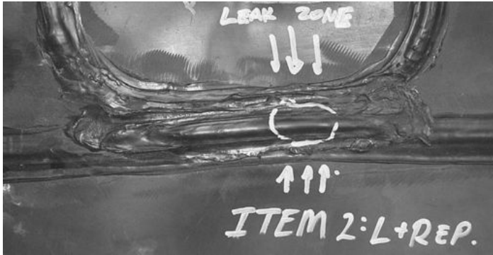
Figure 17.32 Photograph of an example of a poorly made extrusion weld which resulted in a leak zone
