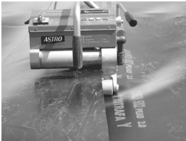
Figure 17.8 Photograph of seaming of HDPE geomembranes liners using a wedge welder (front view). Reproduced by permission of Sotrafa
