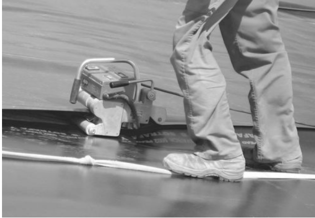
Figure 17.1 Photograph of seaming of HDPE geomembrane liners using a wedge welder (side view). Reproduced by permission of Sotrafa
