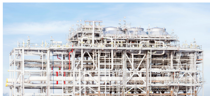
Figure 1. Many LNG assets face an elevated risk of corrosion under insulation (CUI) to develop and proliferate.
