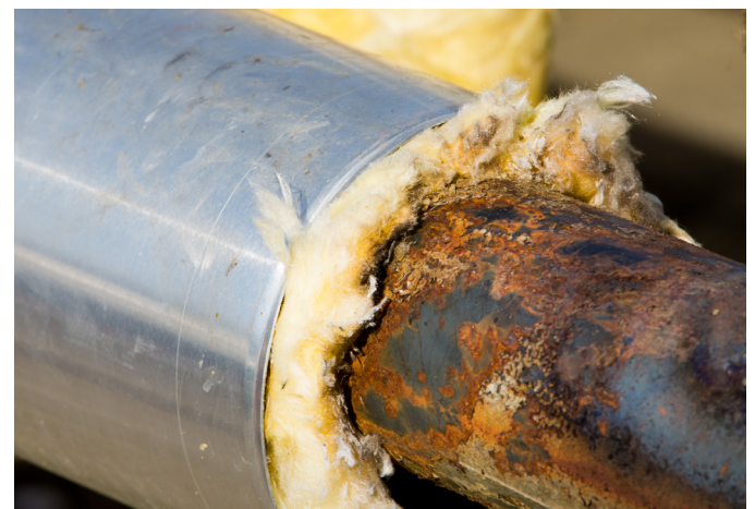
Figure 2. Eating away at steel substrates, CUI may eventually weaken the metal and cause dangerous leaks or explosions to occur.
