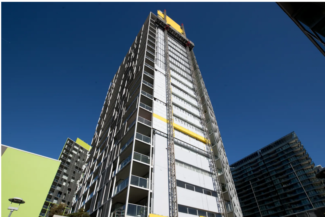
Cladding is removed from the Distillery apartment tower in Pymont. JANIE BARRETT
